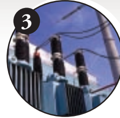
3 At substations, voltage is stepped-down or reduced, to deliver to homes and businesses.
