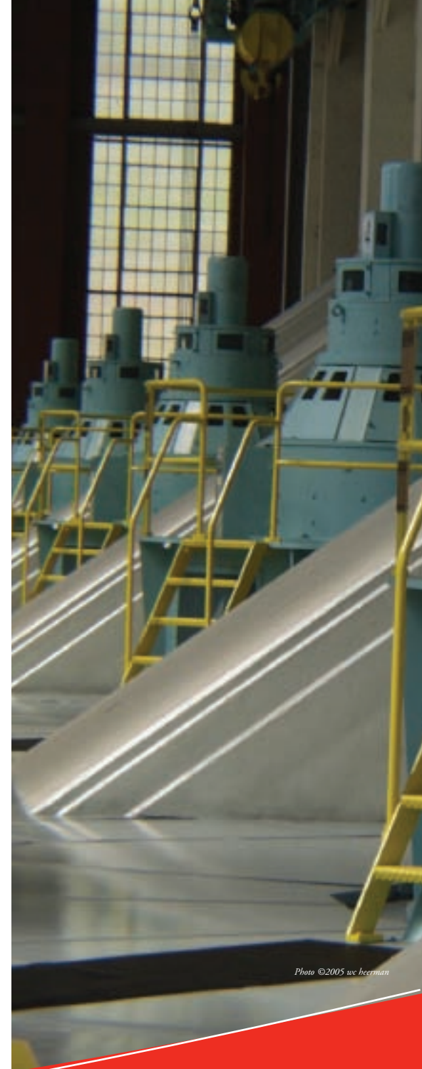
Hydroelectric generators at Lay Dam, near Clanton, Ala.
