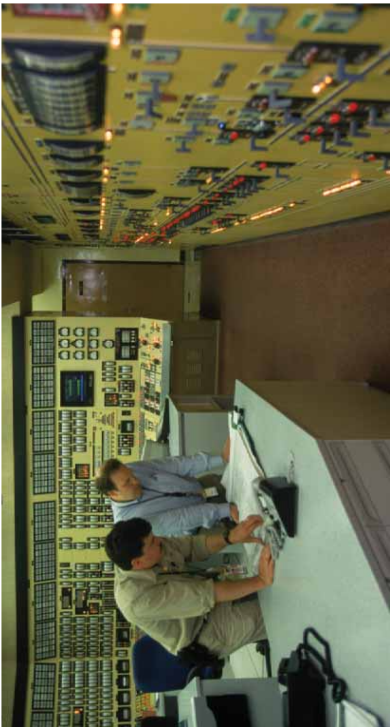
Nuclear Power Plant Control Room
