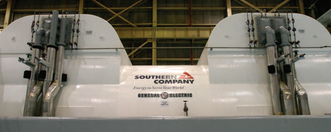
Plant Hatch's Unit 1 Generator
